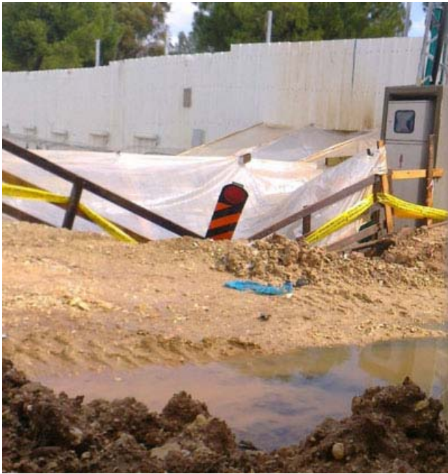
IAA excavation pit inside SWC construction site covered with plastic tarp, supplied with dedicated electrical current for operating heavy machinery and surrounded with warning tape.
