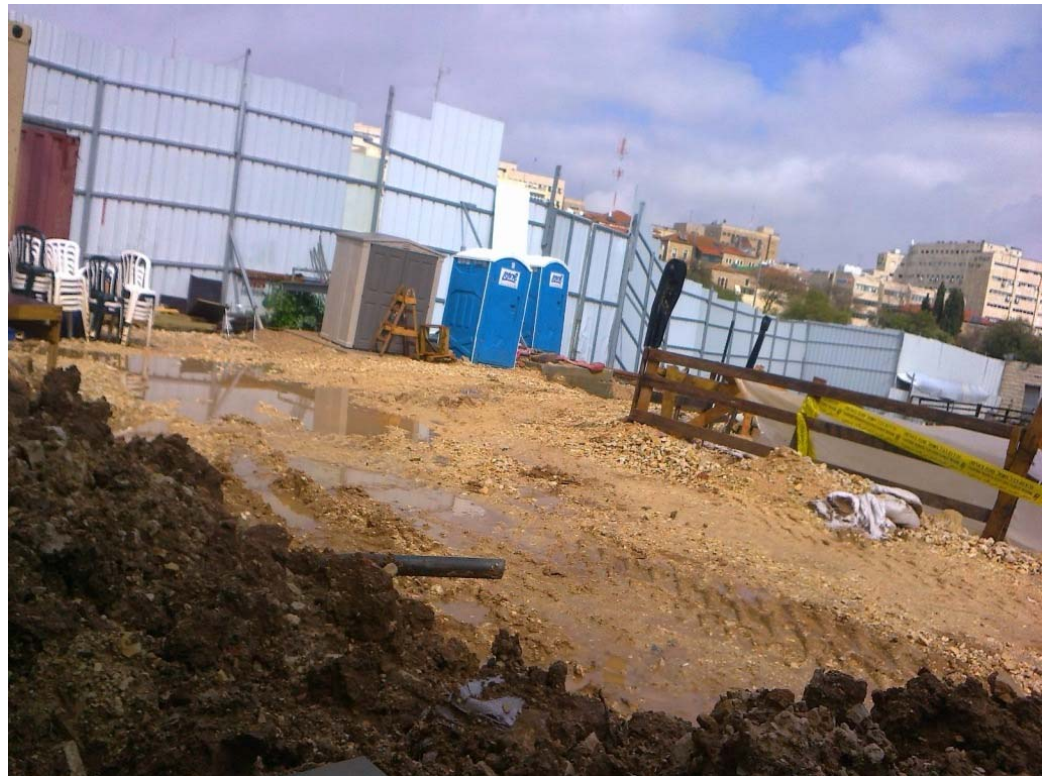
IAA excavation pit inside SWC construction showing inner enclosure wall and portable toilets rented for use by IAA teams onsite
